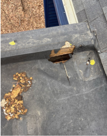
A portion of the damaged roof of Alpha House West
